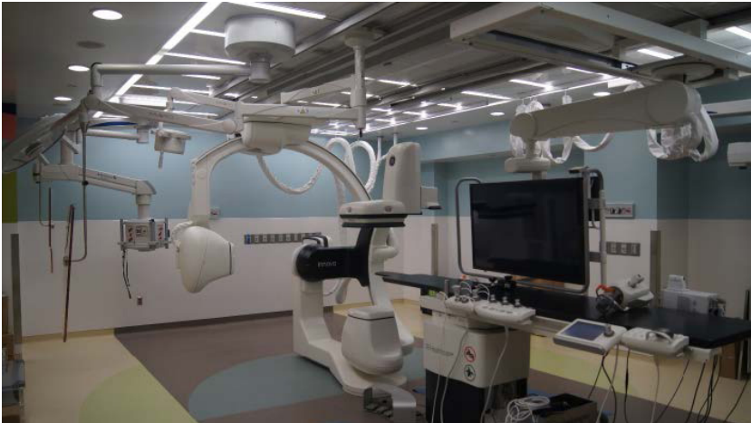
CLEANSUITE ® ceiling system at the VCU Cardiac Catheterization Laboratories.
